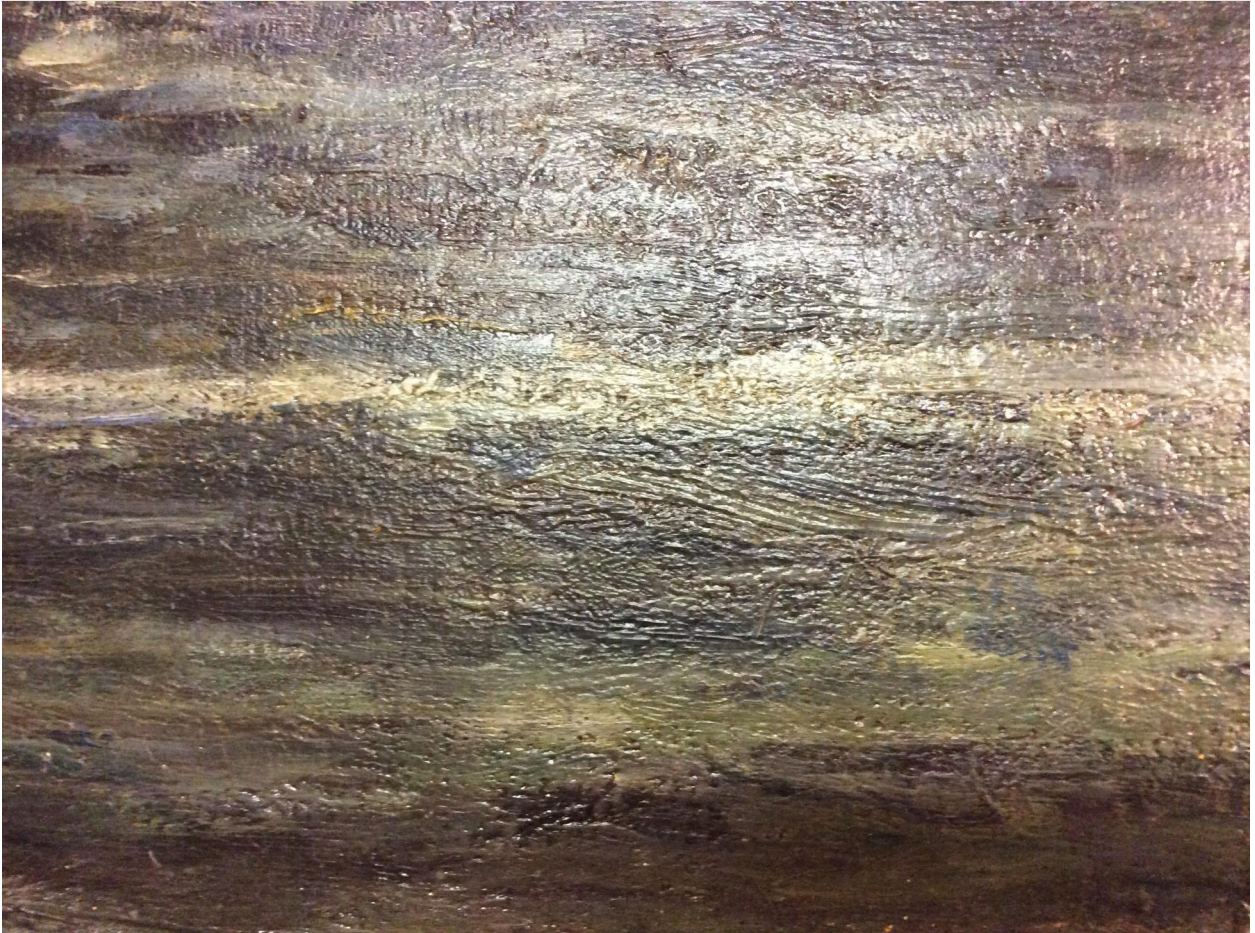
2. Cracking Bottom Left Centre A / Cracks / 11 Aug 2017 / Detail of 1. Overview Front
