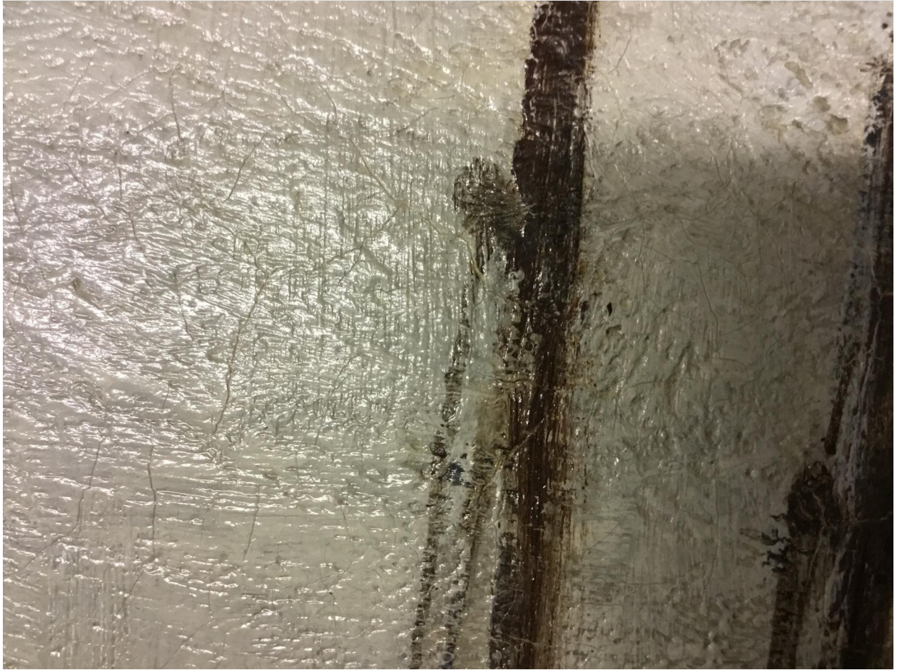
4. Cracking Upper Centre Right C / Cracks / 11 Aug 2017 / Detail of 1. Overview Front
